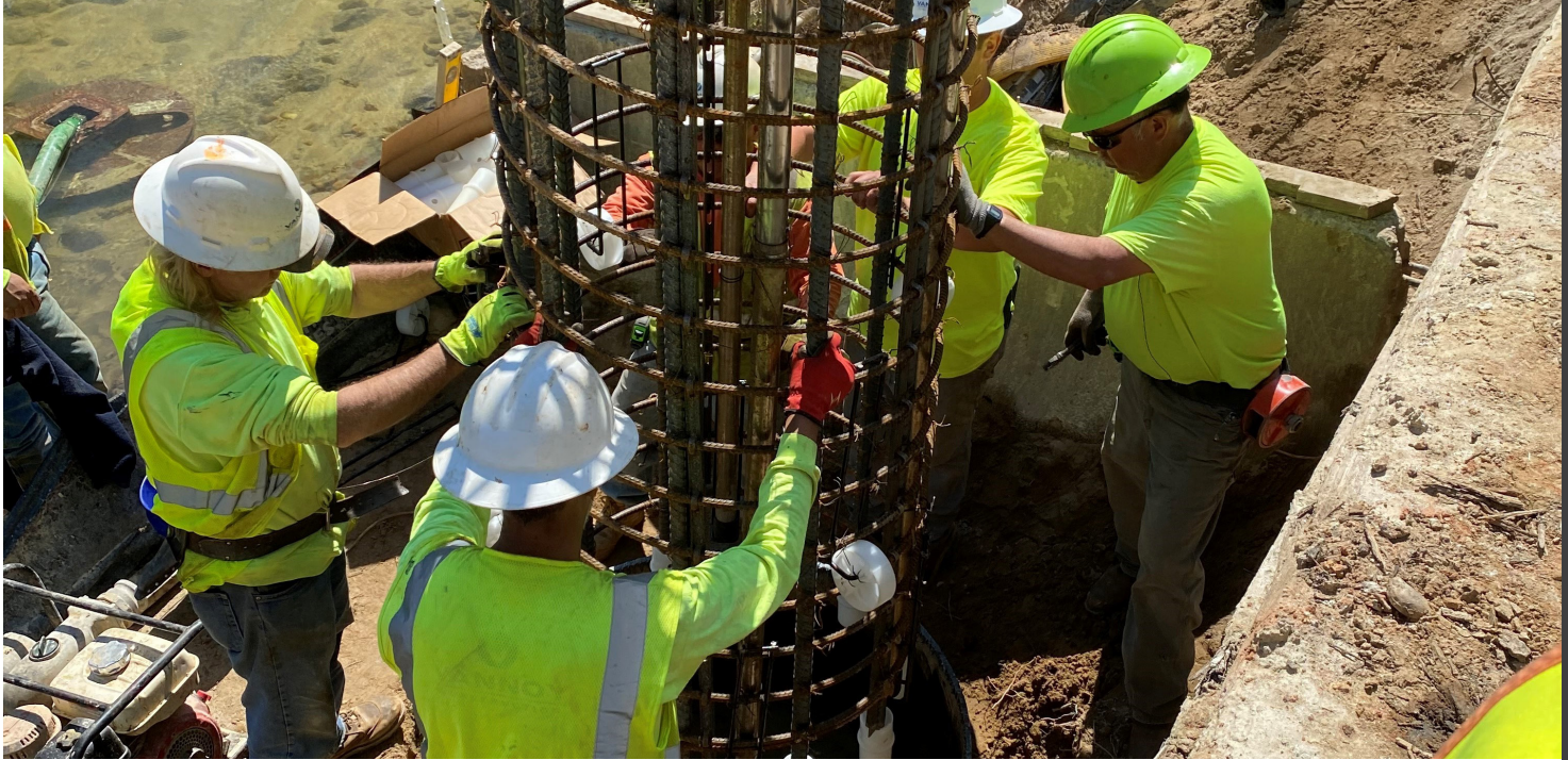
Guiding rebar cage into drilled shaft with Hairpin and ShaftSpacer system attached
