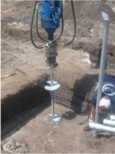
Square shaft lead section installation (back left) Round shaft extension bolted to lead section (right) Square shaft to round shaft transition fitting (front left)
