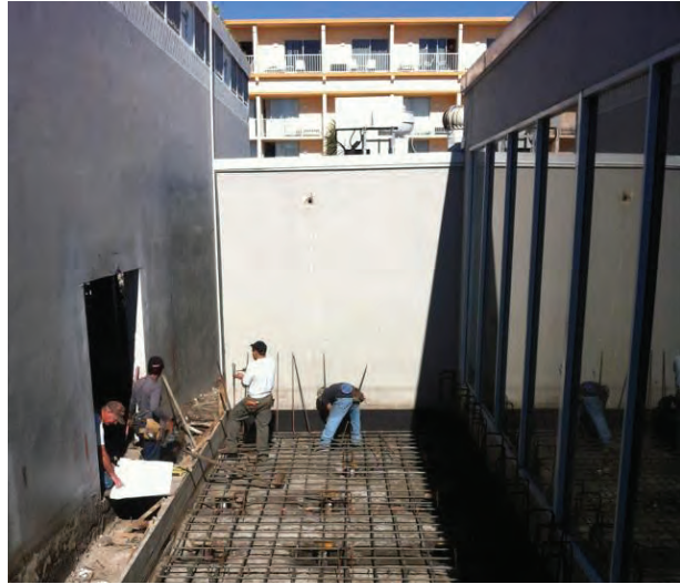
AFTER THE HELICAL PILES ARE INSTALLED AND CAPPED, REBAR IS ADDED FOR REINFORCEMENT PRIOR TO POURING CONCRETE
